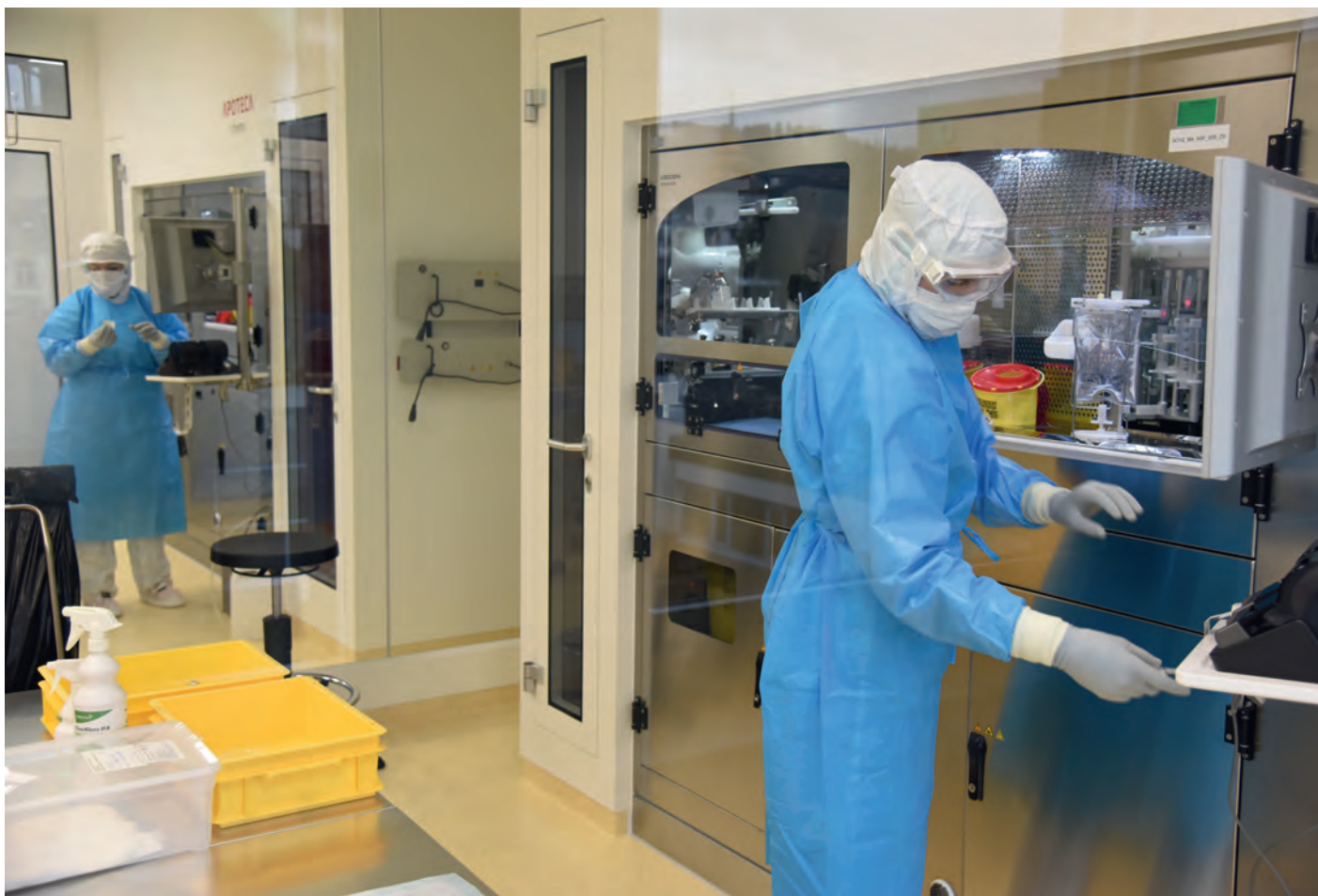
Figure 3: APOTECACHemo installed in Kantonsapotheke Zürich. (Photo Kantonsapotheke Zürich)
